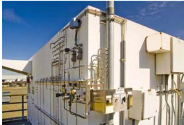
Close-up of tubing/piping (sample gasses, carrier gasses, vent lines, etc.) entering the quality assurance hut
